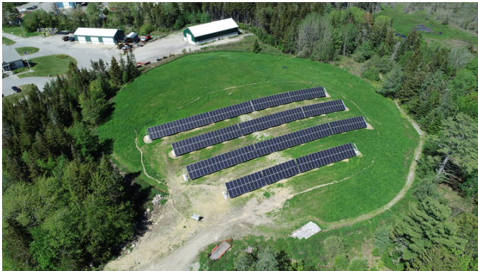
Tremont's municipal array, the first on a capped landfill in our utility's territory.
